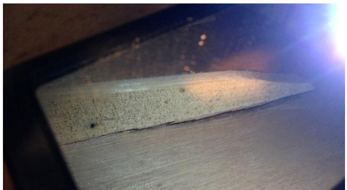
Photo 8: The other brace detached from the top.
